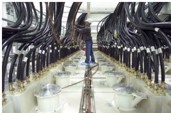
Part of one capacitor bank
